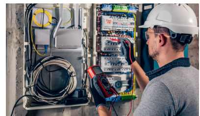
ELECTRICAL SAFETY AUDIT
